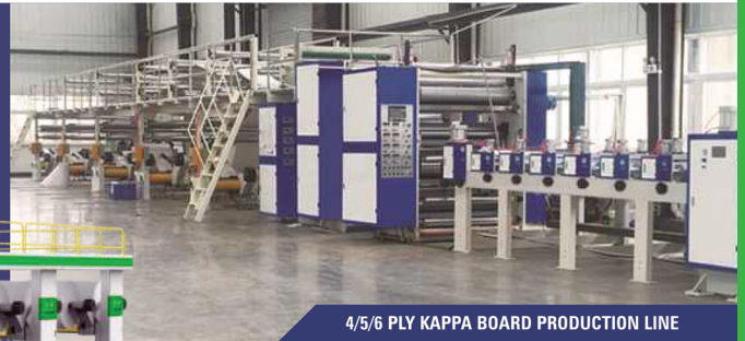
4/5/6 PLY KAPPA BOARD PRODUCTION LINE
